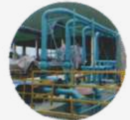
Cooling water pump 冷却水泵
